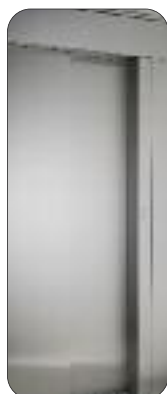
E&I controller panel - closed
