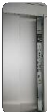
E&I controller panel - open
